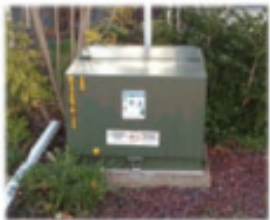
NEW SDG&E Transformer
