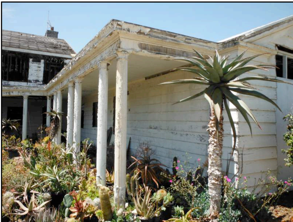
Plate 4.1-6: This photograph of the front north wing structure displays the poor condition of the exterior of Tippet Hall.
