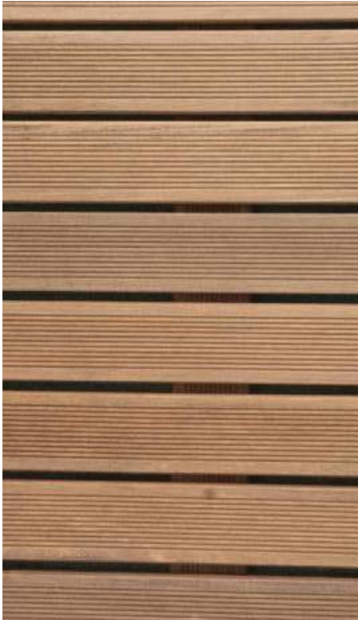
WOOD DECK PAVERS AT TERRACE SOUTH OF TOWN HALL - THERMALLY MODIFIED WOOD
