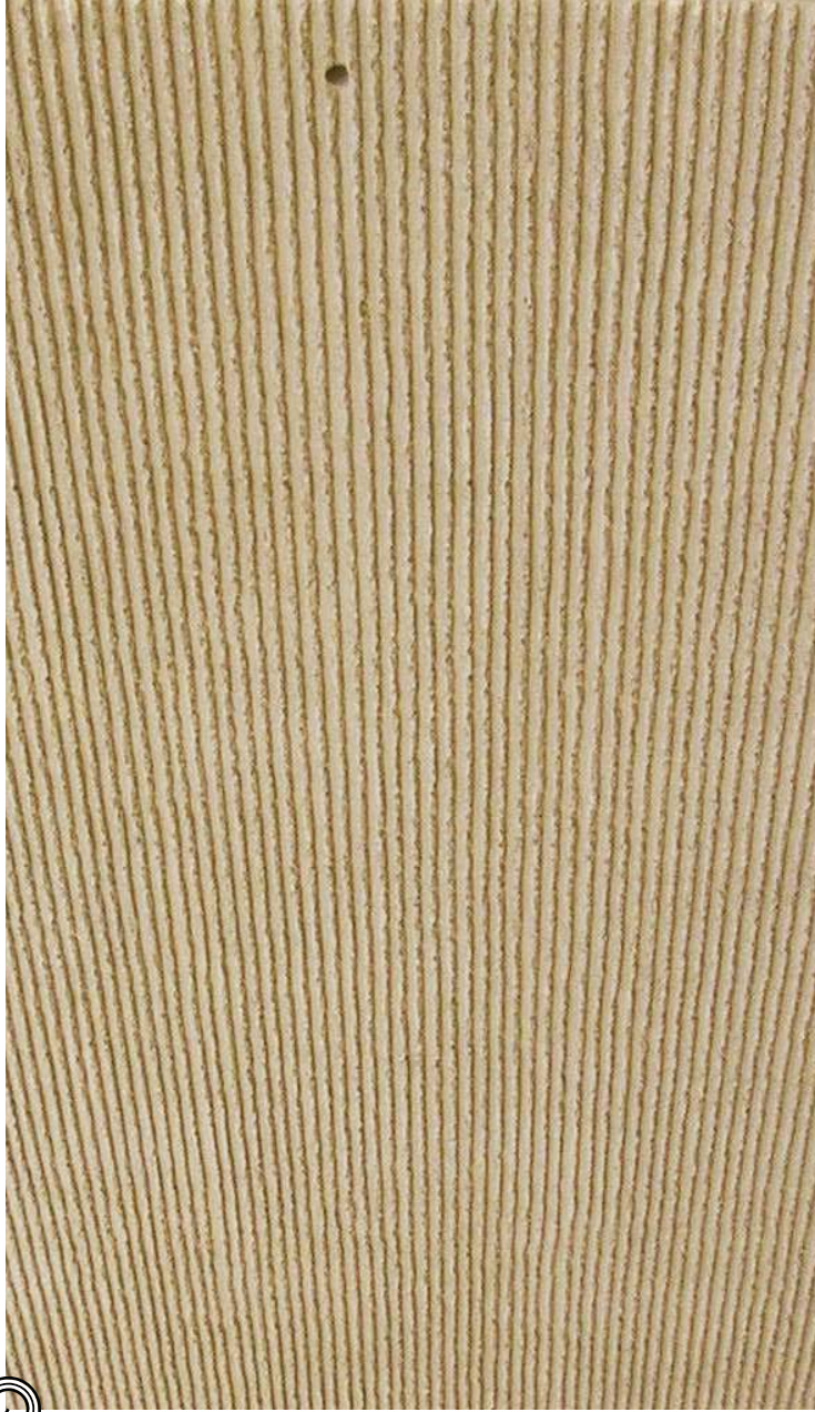
FEATURE SITE WALL ALONG EAST AND SOUTH FACES OF TOWN HALL - ARCHITECTURAL CONCRETE WITH INTEGRAL COLOR, FORM LINER, AND A SANDBLAST FINISH
