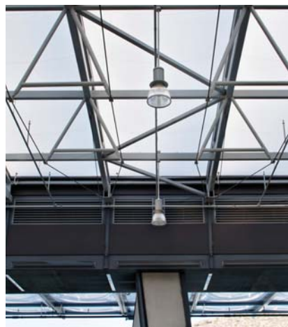
San Ysidro Land Port of Entry: Translucent ETFE pillows reduce the need for daylight.
