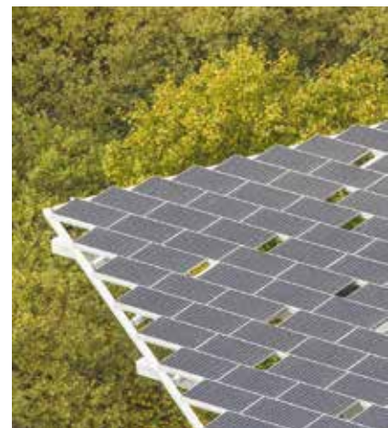
Bullitt Center: Photovoltaic power generation reduces the carbon emissions
