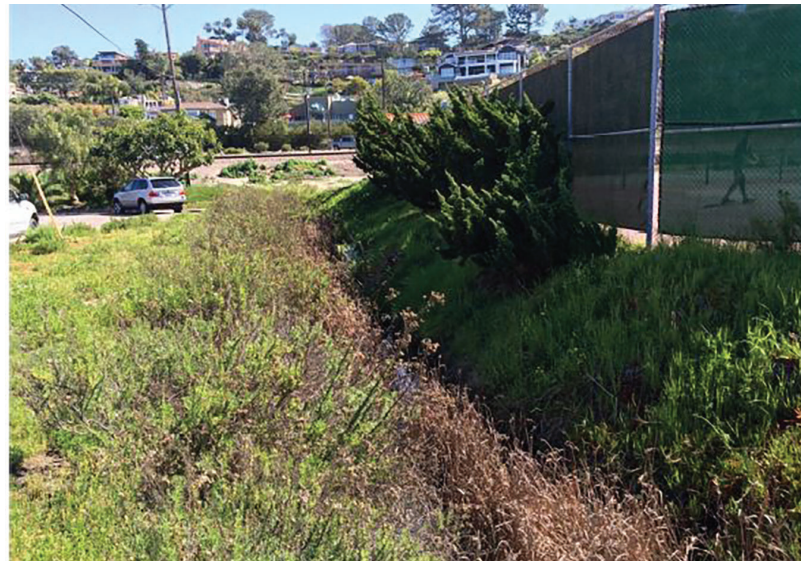
View of drainage feature looking east. Note ornamental juniper along the right bank, chairmaker's bulrush in the middle, and coastal goldenbush along the left bank.
