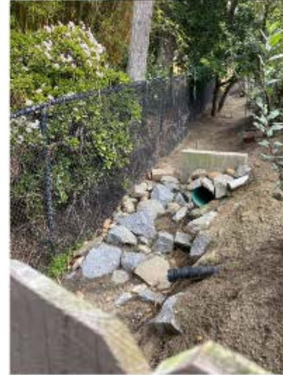
Smith Project open-faced drains installed just above Wilson property (locations marked with red "D")
