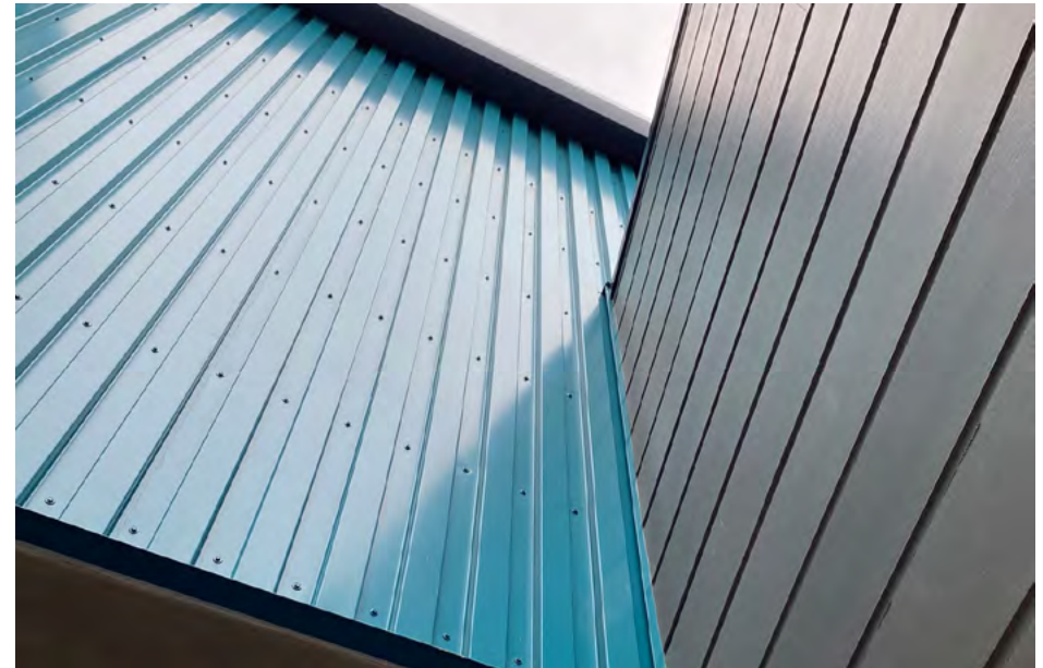
Material change occurring at the inside corner of the plane change.
