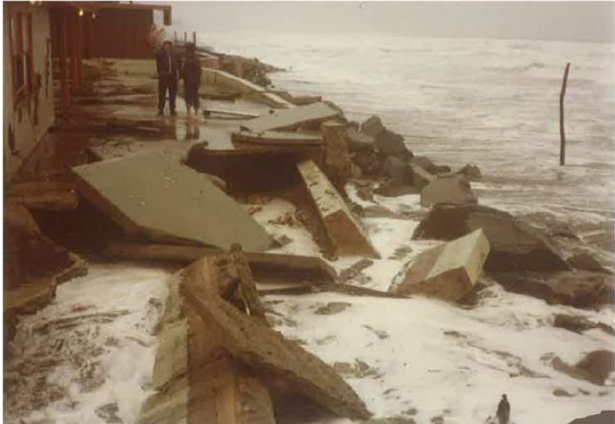
Figure 9.2 Coastal Damage Following 1983 Storm
